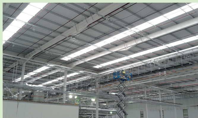
Project: Rolls Royce Advanced Blade Casting Facility Location: Rotherham Product: Zenon Curve & Evolution Liner
